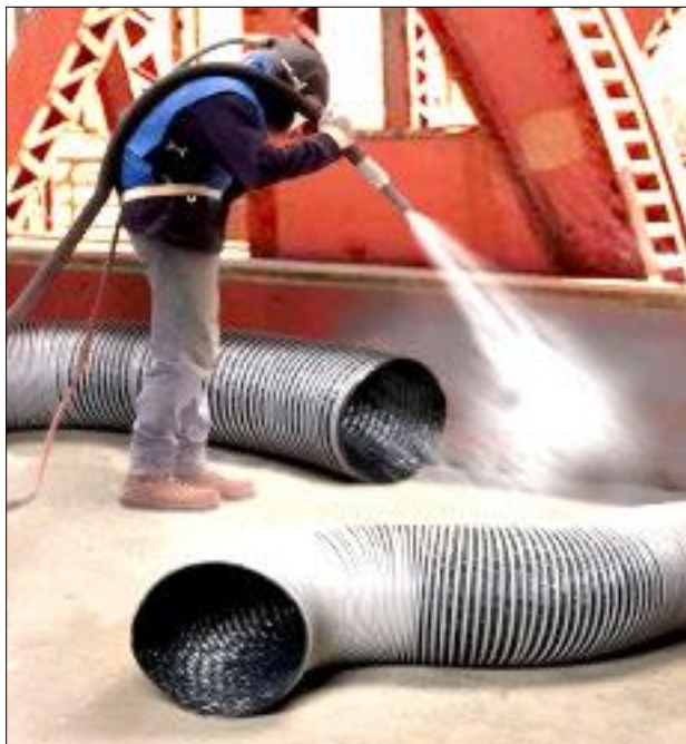
Abrasive blasting using a dust collection system with multiple exhaust ducts. (Photo courtesy of Flexaust, Inc. This equipment is shown for illustrative purposes only and is not intended as an endorsement by OSHA of this company, its products or services.)
