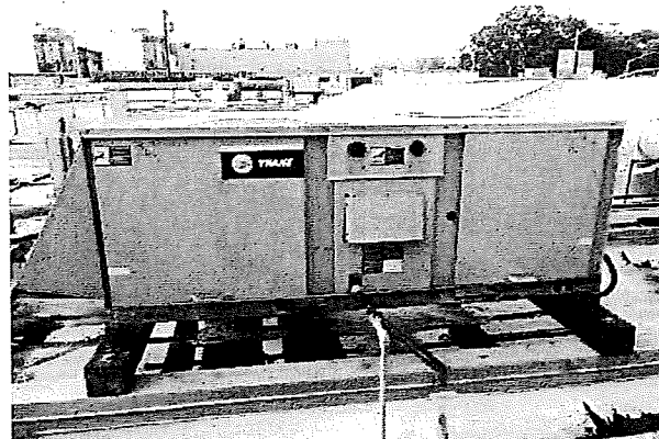
PHOTO #28: Package Unit
