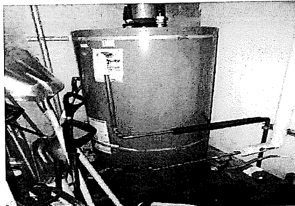
PHOTO #22: Water Heater
