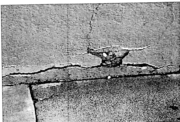
PHOTO #11: Stucco spalling
