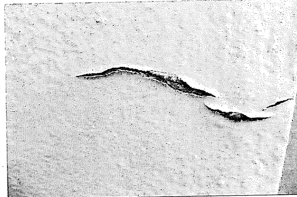
PHOTO #8: Stucco blistering
